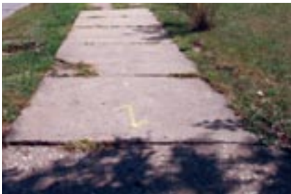
Grass, broken pavement, and heaving surfaces make this sidewalk difficult to maneuver. Photo credit: Dan Burden
